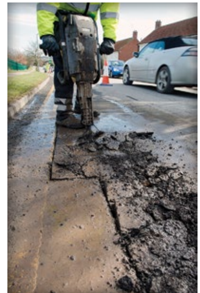
Figure 1. Repairs to utilities are a common sight in cities, incurring costs to cities and taxpayers.
