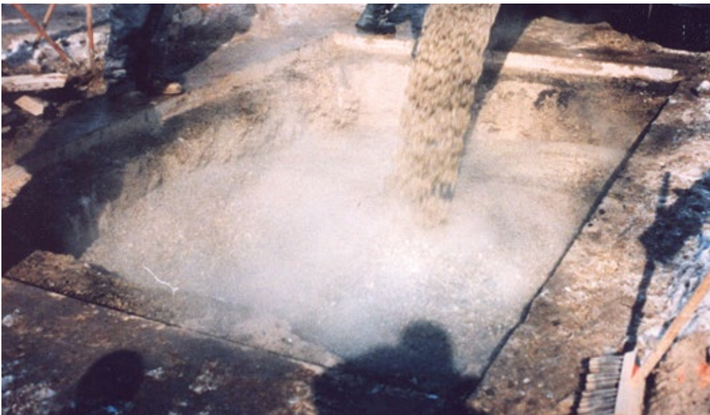
Figure 11. Low density concrete fill (unshrinkable fill) poured into a utility trench from a ready-mix concrete truck.
