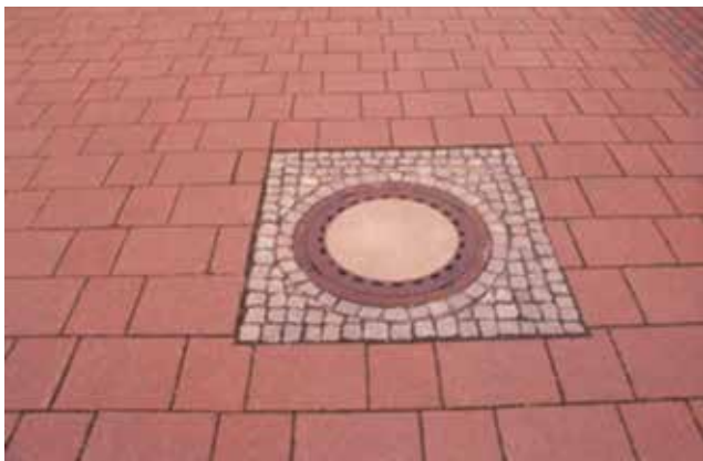
Figure 28. Filling the outside of a utility cover with mortar-set stone paving units
