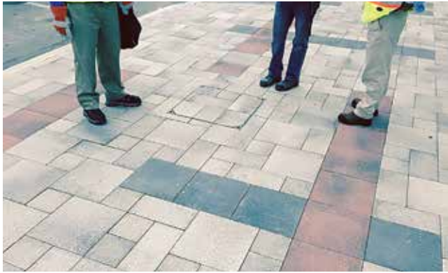
Figure 26. Example of a utility cover that does not fit neatly into the paving pattern.
