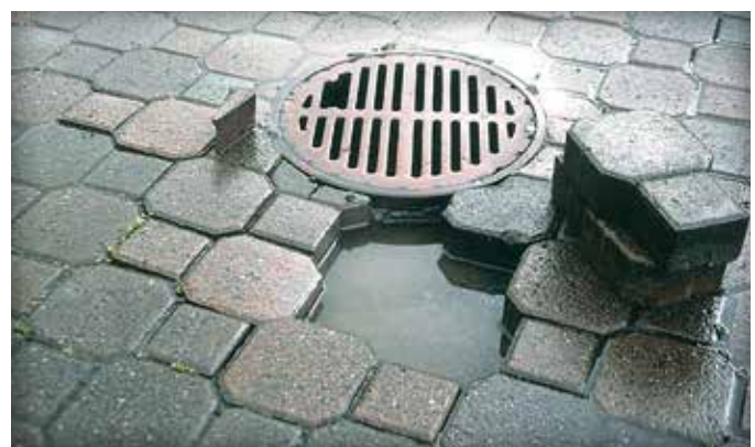
Figure 16. An absence of holes in the sides of this roof drain led to ponding.
