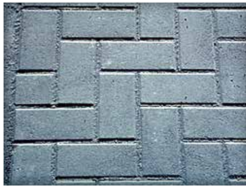
Figure 6. A close-up of the concrete paver surface at the PTI test track.
